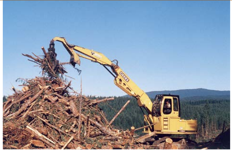
An excavator has the advantage of picking up slash rather than pushing it. It can make taller, more compact piles that burn efficiently, with little soil disturbance.
