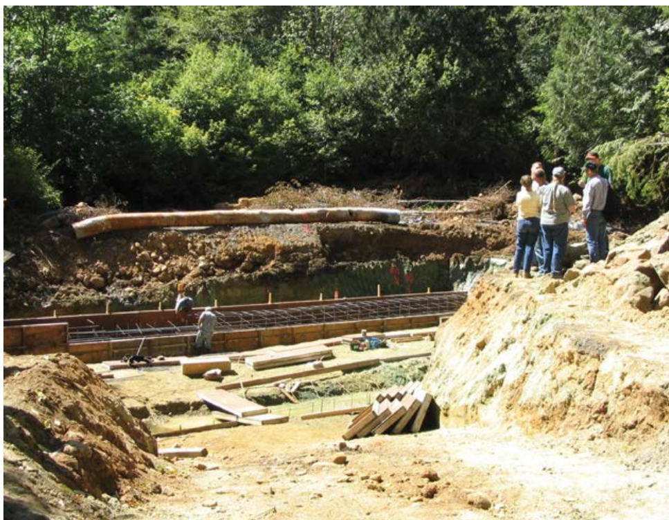
Projects that move a lot of material in or near a stream channel or wetland, such as this stream crossing upgrade, may require a removal-fill permit from the Oregon Dept. of State Lands.
