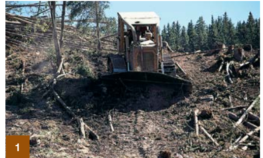
Begin construction of the skid trail cross ditch at the far edge of the skid trail.
