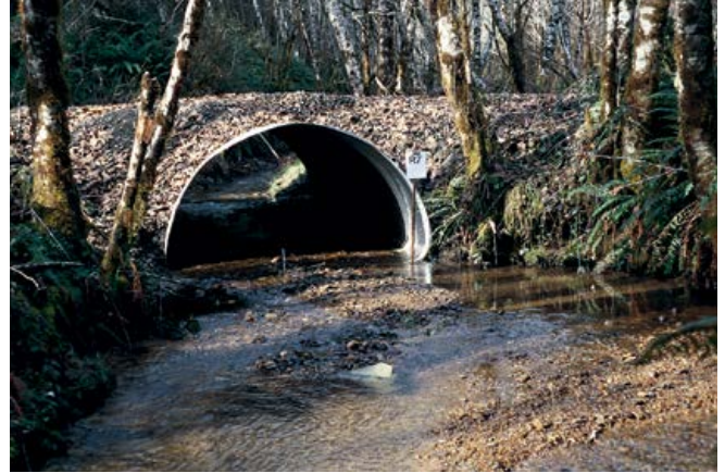
Arch culvert on a low clearance road, sunk into the streambed to allow for fish passage.
