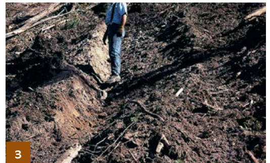
The finished skid trail cross ditch should be deep. This is more than a water bar.
