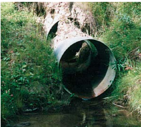
Watch for damaged culverts that need replacement. Repair work should be completed during dry weather.
