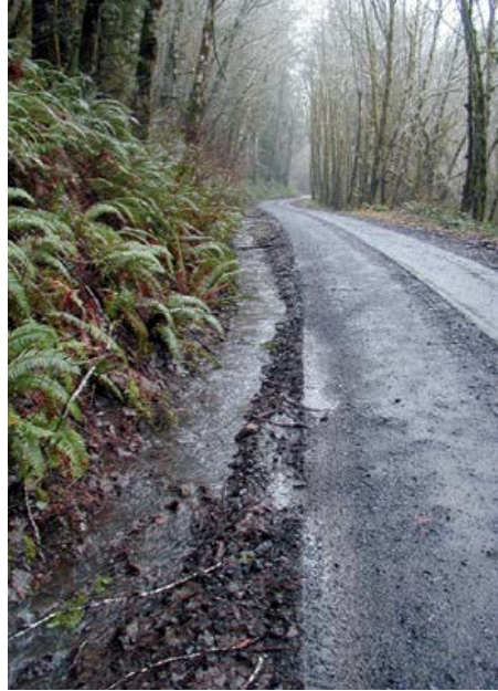
Durable rock surface on a log hauling road during heavy rain. Notice that the water in the ditch is clean.
