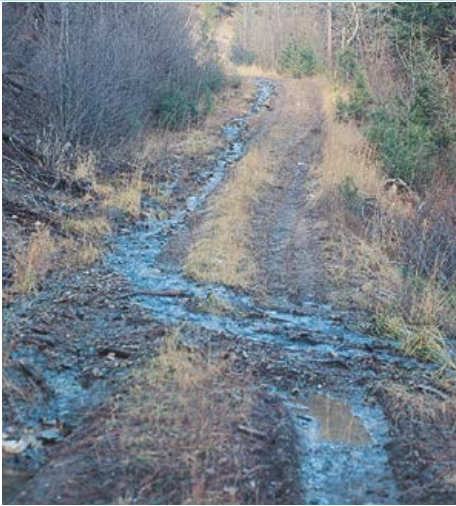
Not a major sediment problem yet, but when roads become channels for drainage, major sediment pollution can result
