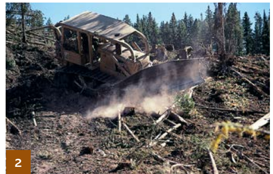
Cut an extra-deep cross ditch at an angle greater than perpendicular to the skid trail, and be sure the ditch is open so water can drain out.
