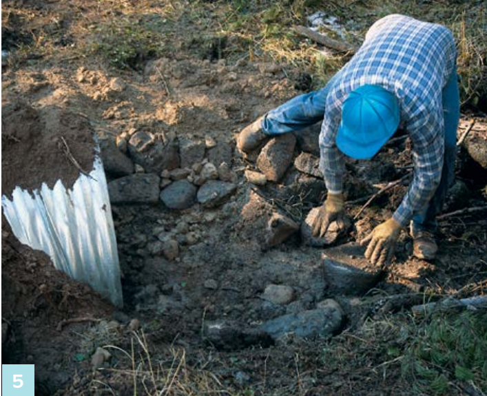
5 Armor the culvert inlet and outlet. Rocks, logs or grass seeding can be used to protect these locations against erosion. Check the area upstream and downstream from the culvert. Clear the upstream area of woody debris that might plug the culvert.
