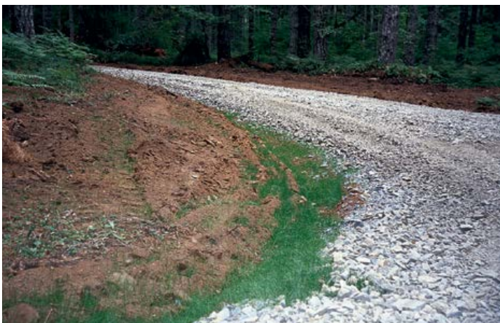
Road surfacing can double the cost of a road. However, gravel roads can provide all-weather access, reduce road maintenance costs and protect water quality by covering the soil with a weather-resistant surface.
