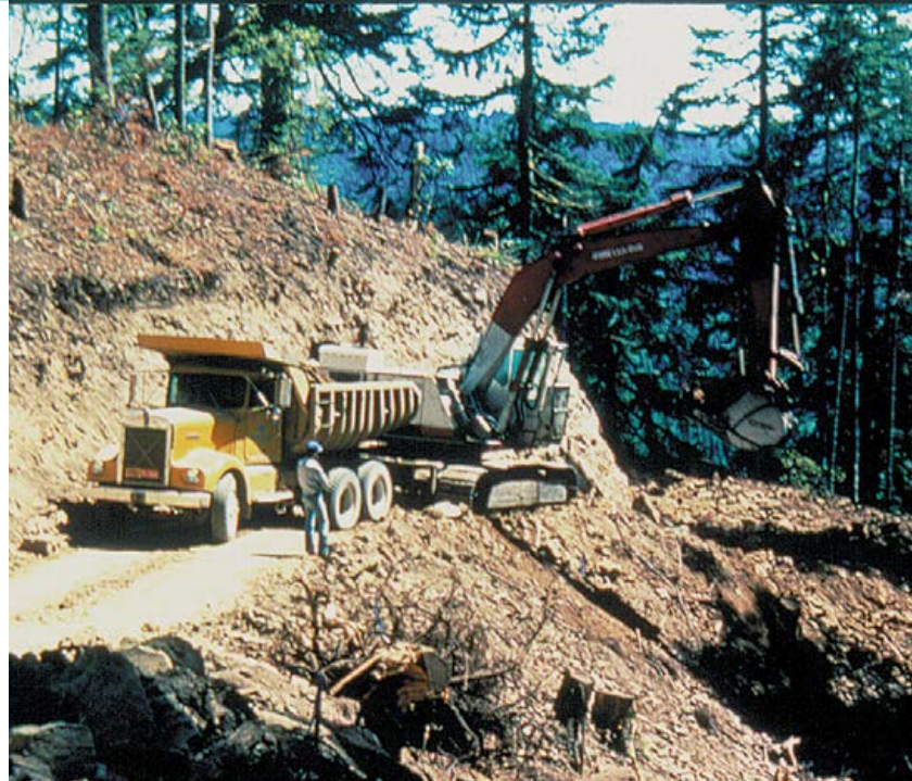
When constructing a full-bench road, the entire road surface is excavated in the hill. The excavated material is end-hauled, meaning the material is removed by truck to an area needing fill or to a stable disposal area.
