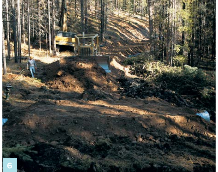
6 The road approach to the new culvert is the next phase of construction. Be sure that the culvert fill above the top of the pipe is at least 18 to 24 inches, to protect the pipe from damage by traffic.
